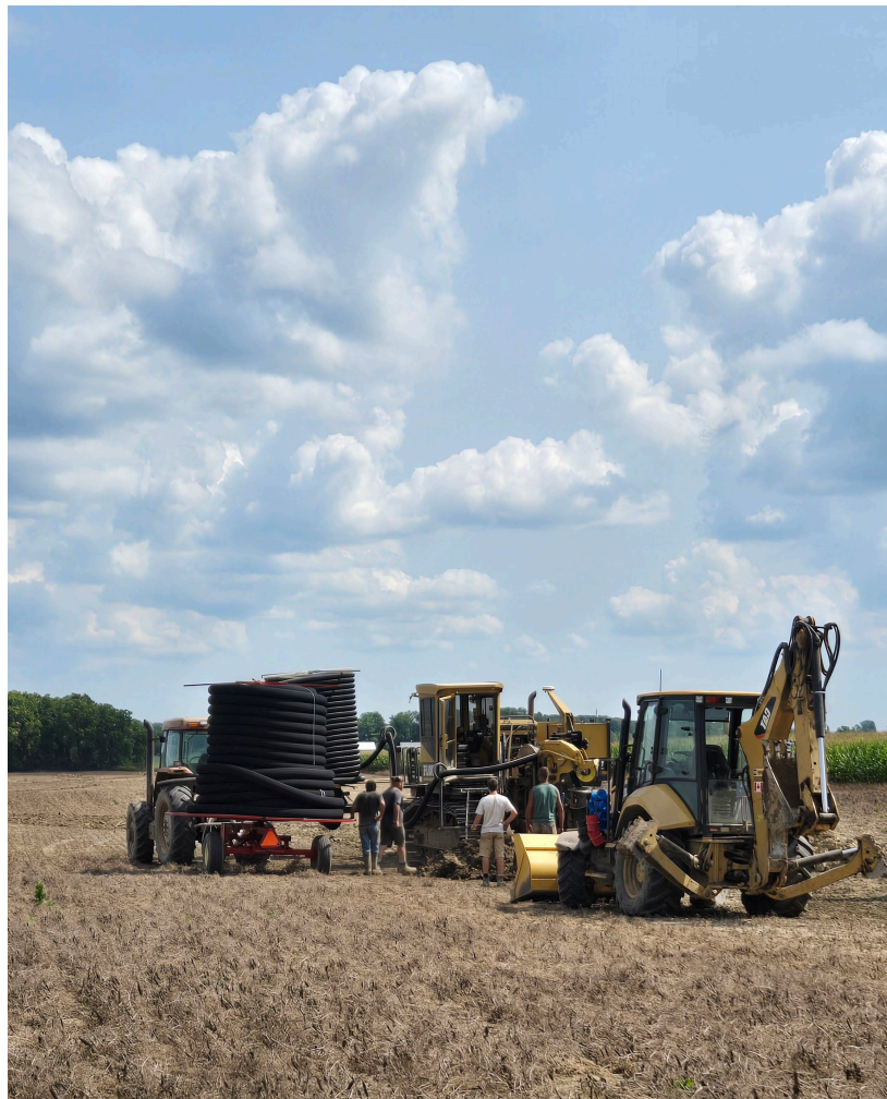
Figure 9. Tiling being installed in a field near Mt. Brydges, Ontario. Photo from FAS on August 13, 2024.
